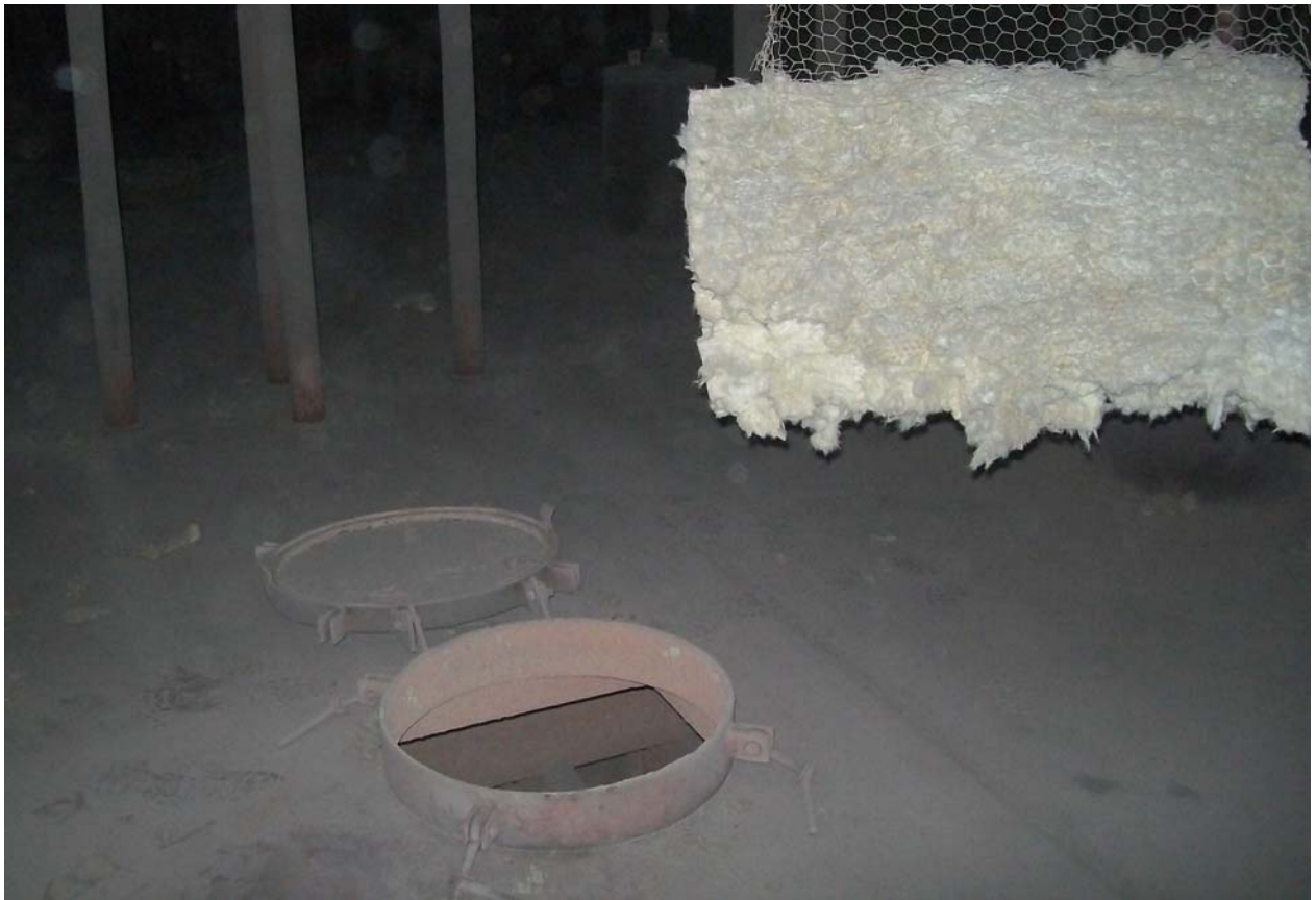
Photo 13: In this case, the inspection door was left open in the penthouse. The ID fan has draft has led to falling of mattress from roof.
