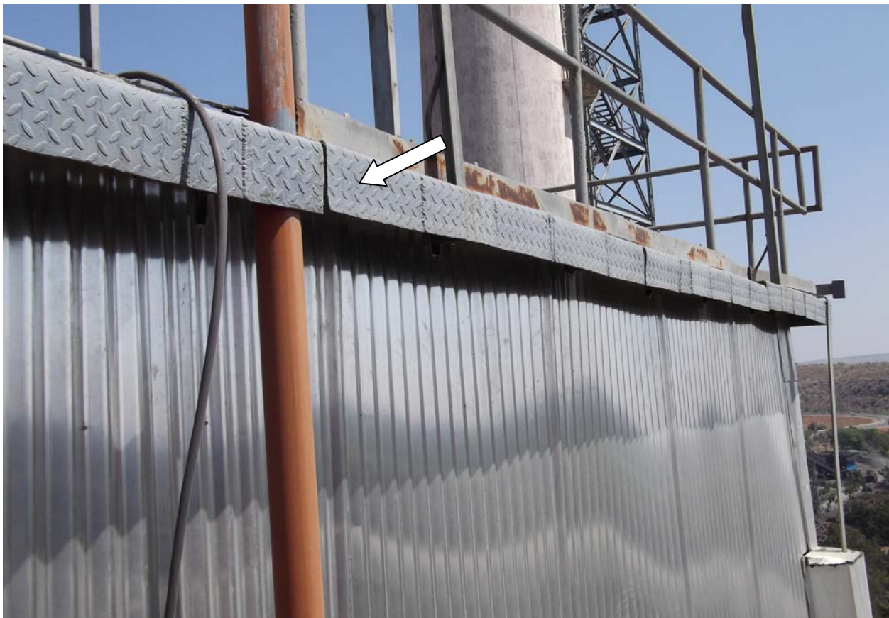
Photo 15: This the way the rain water ingress in to insulation is prevented. Yet the skipped welds can cause water running in to insulation.
