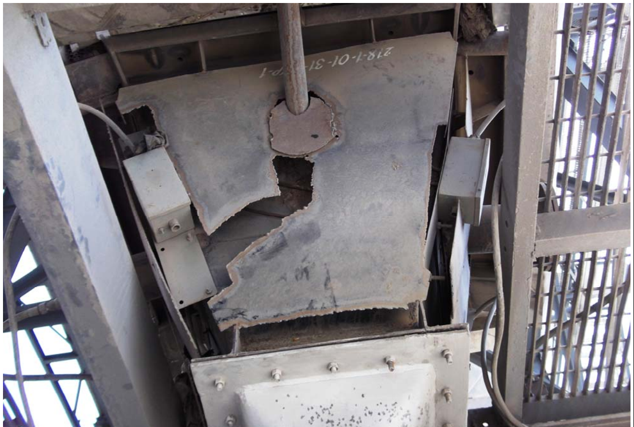
Photo 23: The hopper heaters installed by an ESP supplier without the purpose. The box should be completely sealed and insulated outside to help ash flow.
