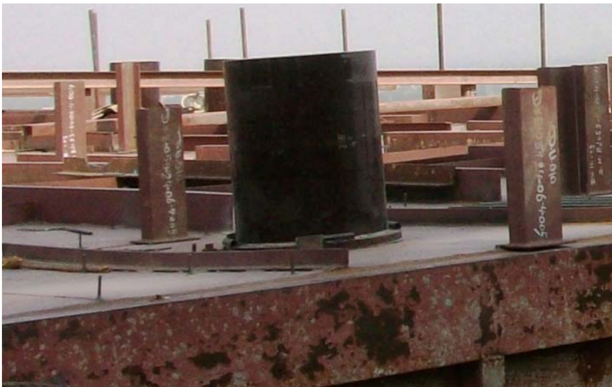
Photo 20: Improper base for insulator, which supports the emitting frame. Such defects leads to insulator break down.
