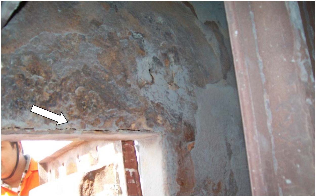
Photo 3: Incomplete welding of inspection door frame and absence of double door system is seen causing corrosion of ESP casing.
