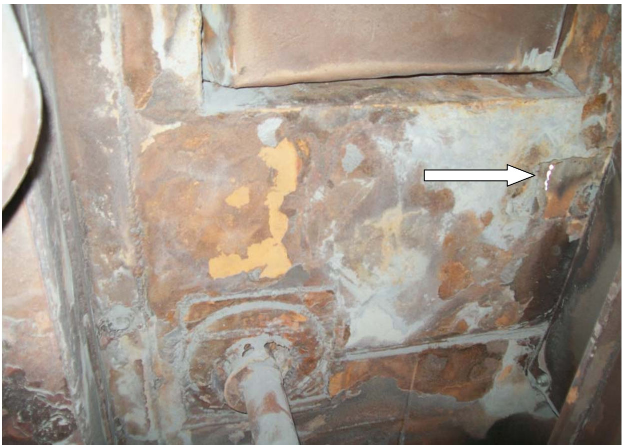
Photo 7: Condensation of flue gas inside ESP casing when the casing is exposed to heat dissipation by improper insulation.
