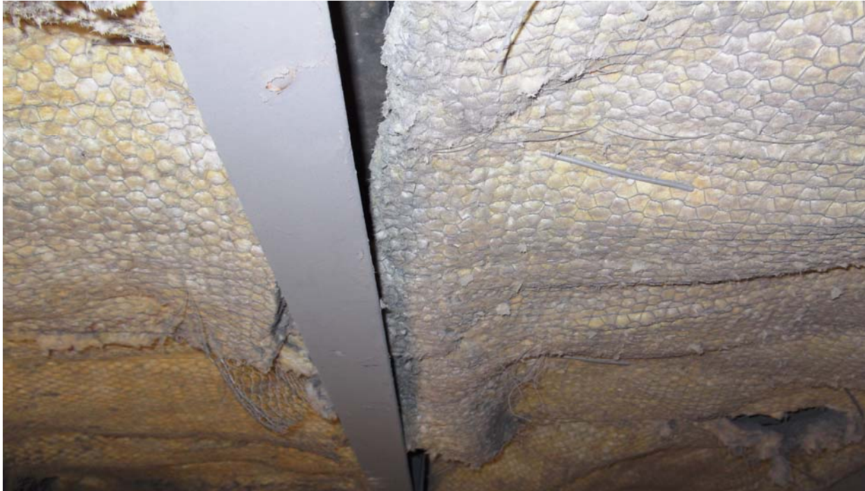
Photo 11: The incomplete penthouse roof insulation is seen here. Patch insulation is not the right way for any hot surface.
