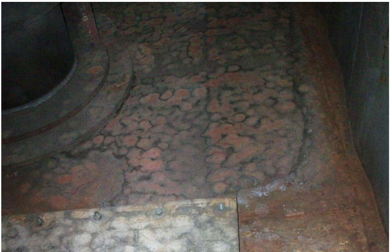
Photo 9: Condensation of flue gas inside the penthouse. When the boiler frequently stopped for some reason, the condensation of penthouse is unavoidable. If there is any door open at penthouse, the flue gas fills penthouse and starts condensing.
