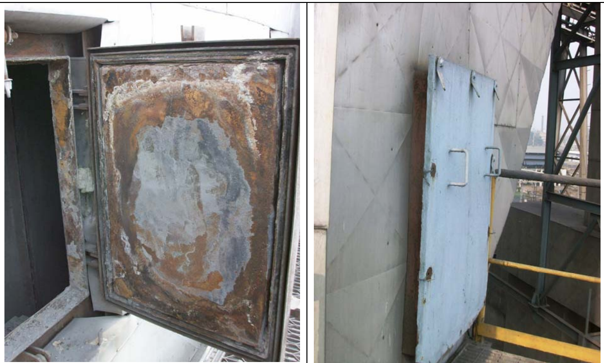
Photo 4 & 5: ESPs are to be provided with a double door system. This ensures that there is no exposed uninsulated area around the door. In the absence of double door system, the corrosion of casing is more. These problems are addressed by double door system. The photo at right is the arrangement with double door system. In double door system placement of LRB mattress can help to keep the inner door warmer.
