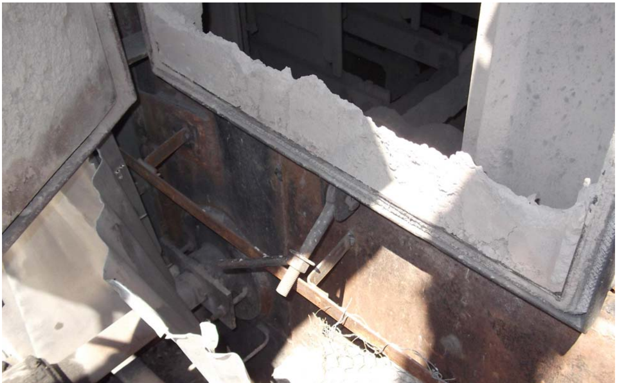
Photo 6: This is the area below inspection doors. In most ESP this will be the case. The ESP casing is exposed to ambient. After some time, the casing is seen punctured.
