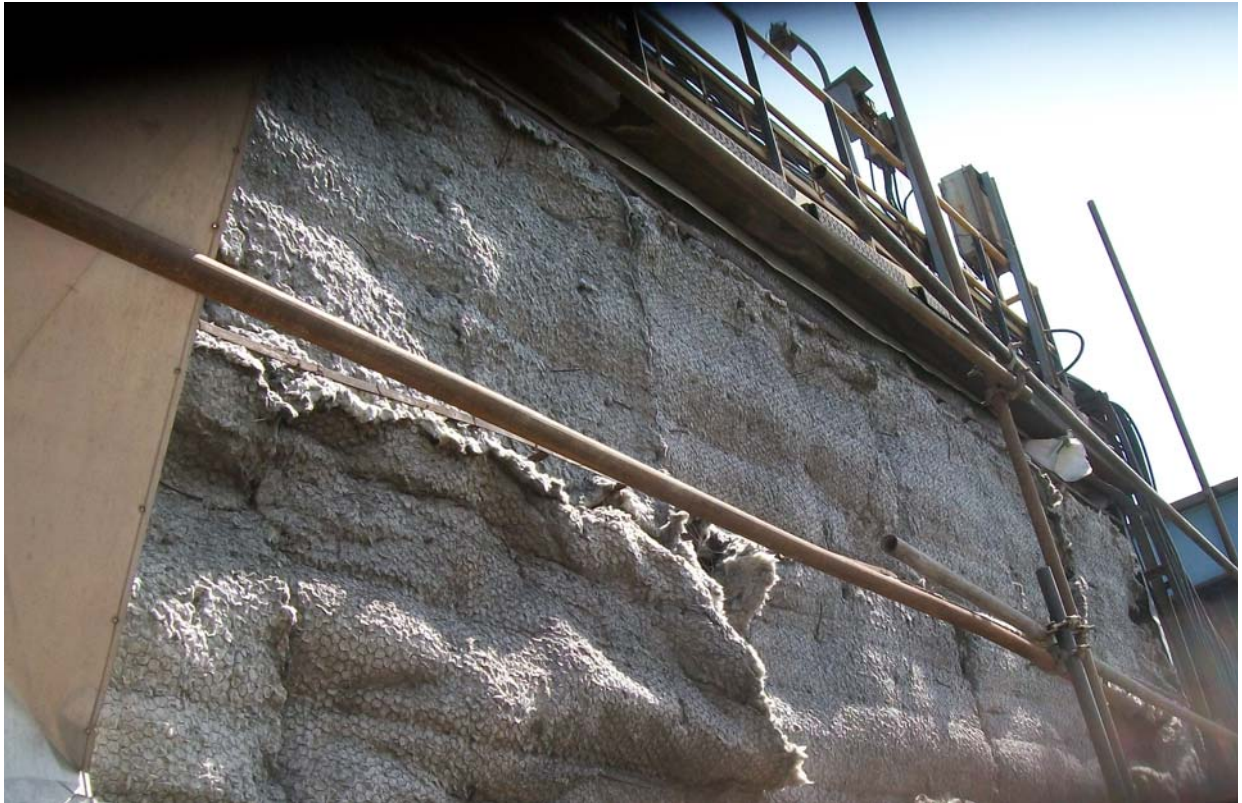
Photo 18: The insulation mattresses have to be properly overlapped. In case there is localized cladding disturbance, the cladding needs to be attended on priority.
