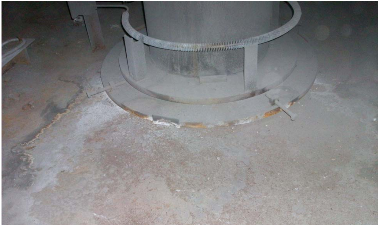
Photo 22: Water pools with ash are seen in ESP penthouse. This space is supposed to be a clean space. It proves there is no perfect sealing between ESP inside and the penthouse. Water around the insulator is unsafe.
