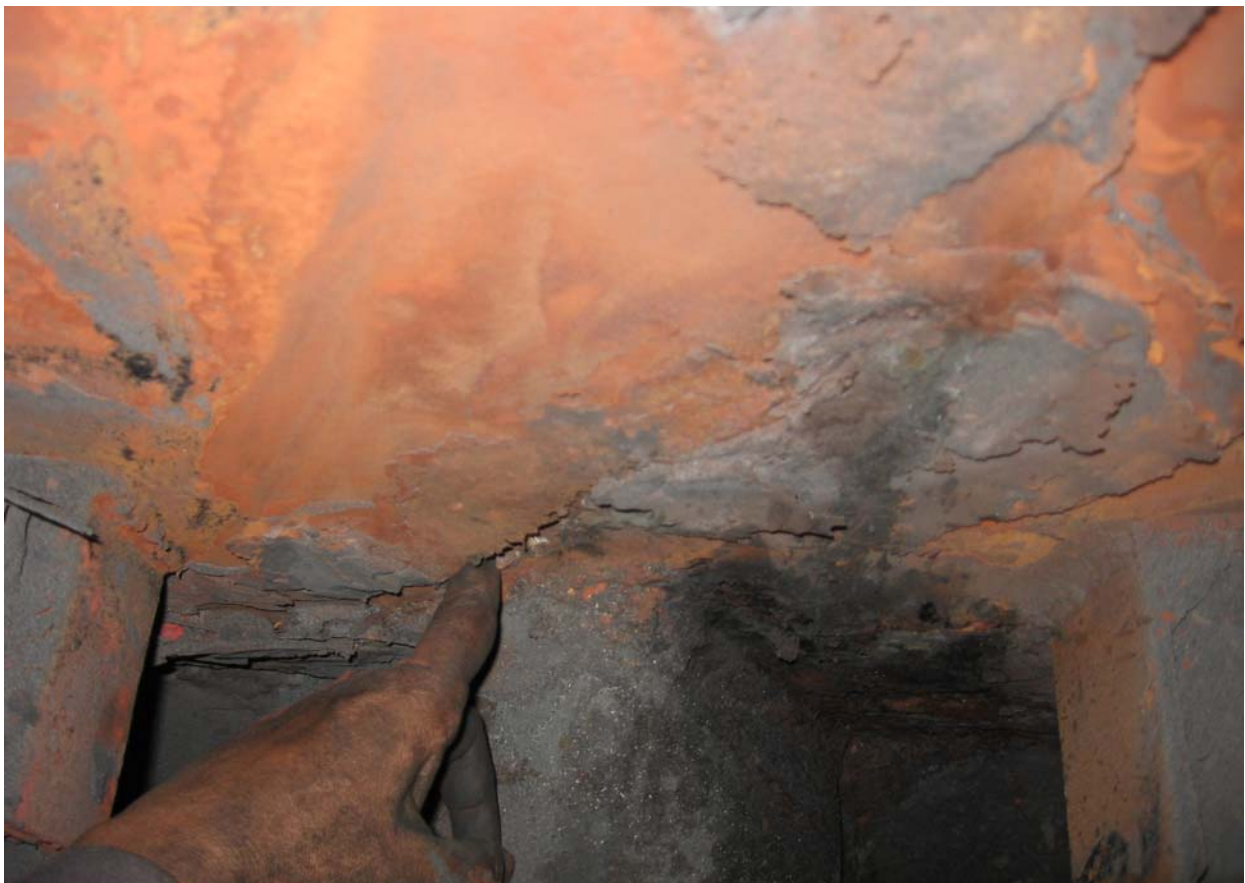
Photo 17: The casing in the above case developed holes and led to more air ingress ultimately affecting the steam generation rate. This is in the case where the columns were not insulated.
