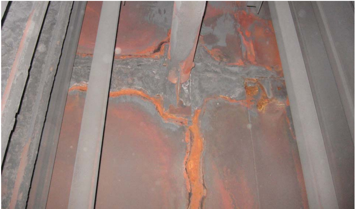
Photo 16: The ESP casing seen damaged in a plant where the main column & tie beams were not insulated. Hence the ESP collapsed in two years time.
