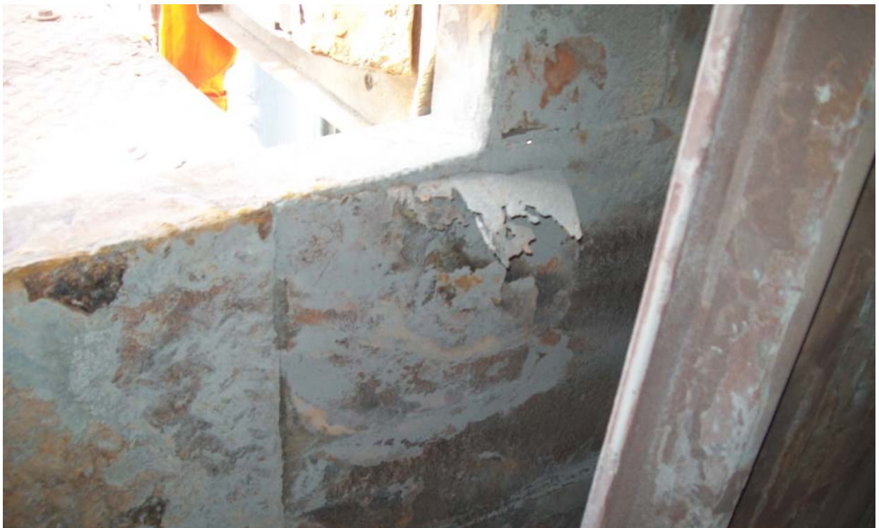
Photo 2: Condensation of flue gas below the inspection door. The door is not a double door system.
