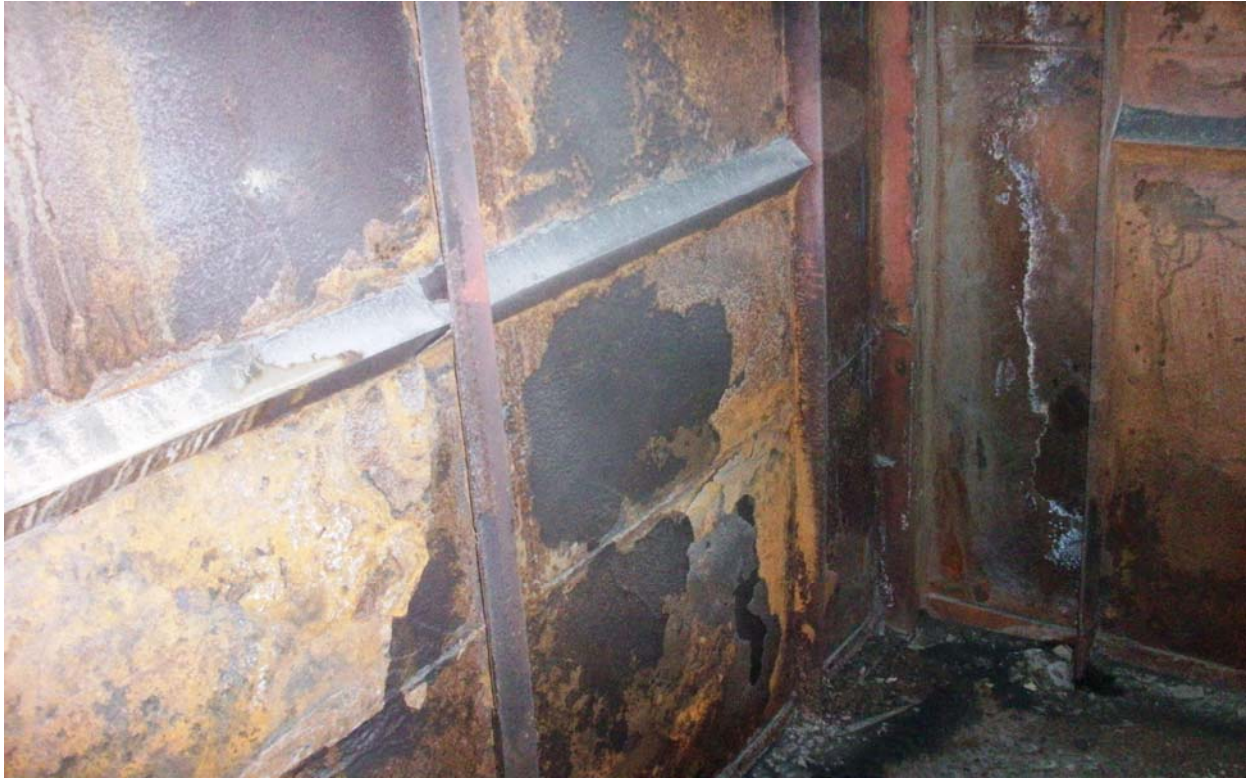
Photo 12: Rain water running down inside the penthouse, due to incomplete sealing at top.
