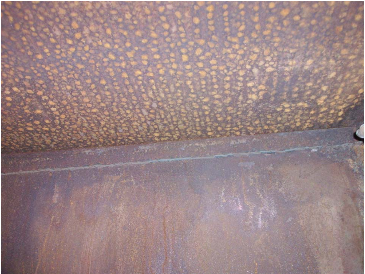
Photo 10: Condensation of gas from ESP penthouse roof plate. No insulation is provided by the manufacturer.
