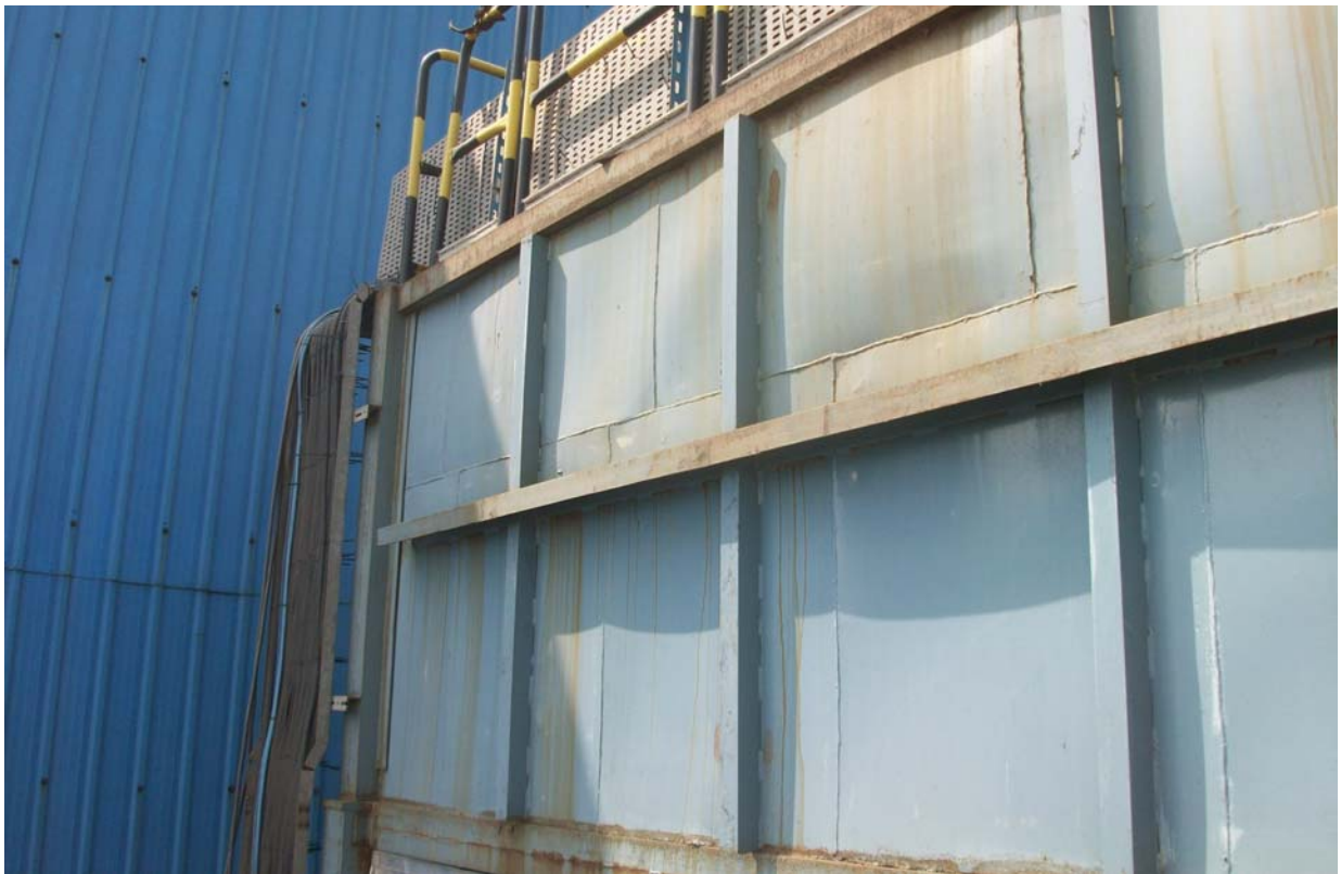
Photo 8: The penthouse is seen uninsulated by an EPC company in to manufacturing ESP.
