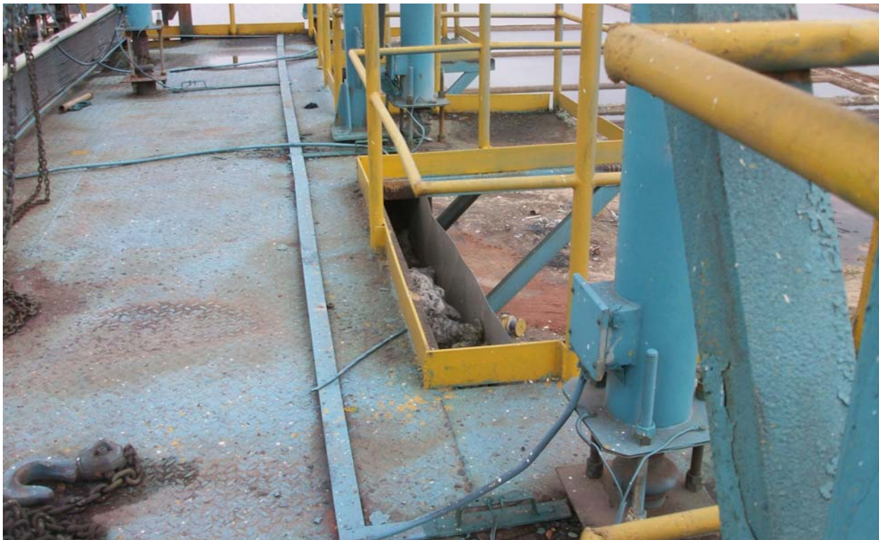
Photo 14: Improper roof of ESP. The rain water enters inside the ESP insulation. This leads to gas condensation and after some time, the casing starts failing.
